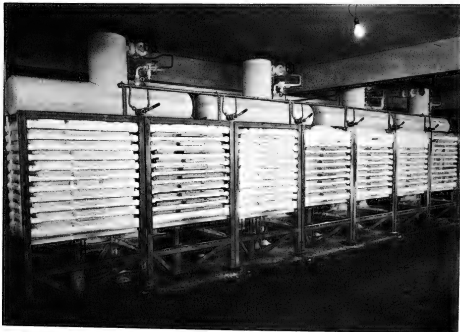
Plate-freezing equipment in a modern Icelandic fillet plant.
